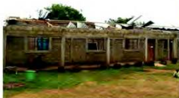
Storm Damage to roof at Matsatse in December
